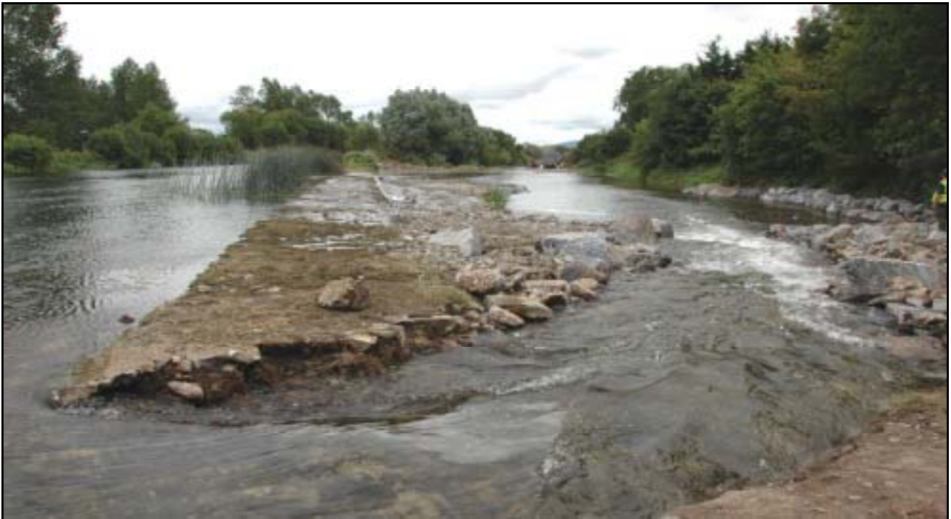
A photograph of the new fish pass at Ballyellen Weir (Photo courtesy of Alan Cullagh, SRFB)
